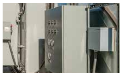
Rooftop Control Systems
